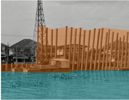
FIG. 13 (Top) River floodwall being heightened in Nonthaburi area, segmenting riverfront lives and water
