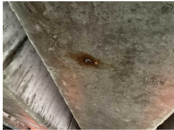
(b) Beam 6 bottom face.
