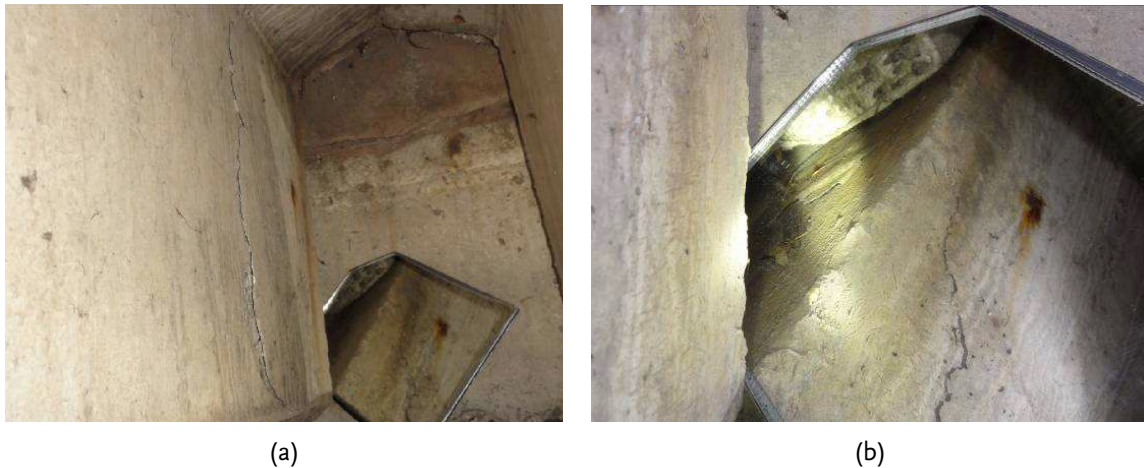
Figure 3.8: Damage to beam head (a) and cone (b) of beam 13 in 2011.
