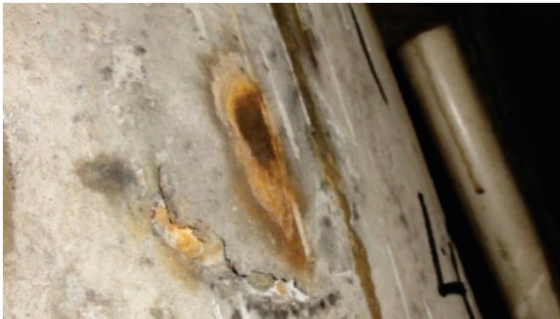
Figure 3.1: Example of a cone with corrosion damage (C4).
