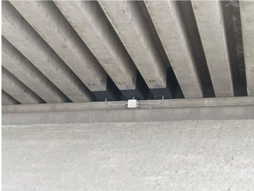
Figure 3.7: The cast 3+ composite anode system applied to beams 12, 13 and 14 of STP01 on the Sluinerweg viaduct.
