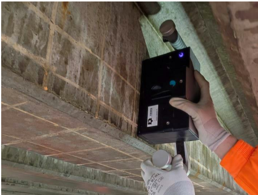
Figure 2.15: Proceq Pundit PD8050 UPE device used for inspecting tendon ducts after the localisation of the reinforcement with GPR.
