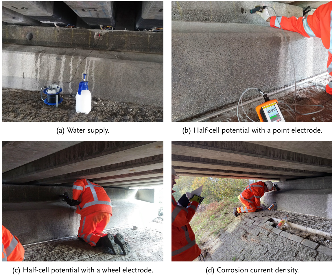
Figure 4.8: Corrosion measurements on the support beam.
