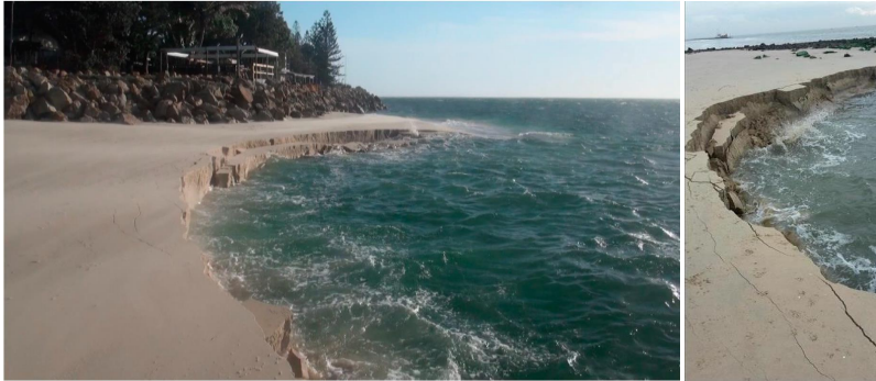
Figure 1.3: Ongoing breaching flow slides: Amity Point captured on 18 August 2014 ( left ), Ameland Island Southwest, the Netherlands, 2017 ( right ) ( Mastbergen et al., 2019 ).
